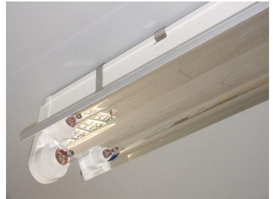
armature with reflector and UV lamp
