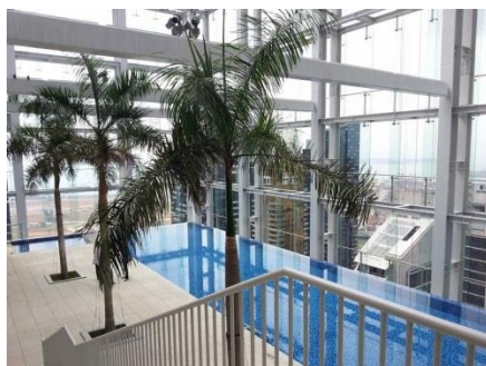
UV treatment for a public swimming pool on the 37th floor overlooking the Singapore skyline and harbour
