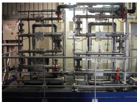
UV treatment for water preparation for CSB reduction at the Hamburg Dock
