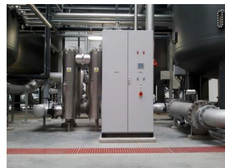
UV treatment for water preparation in Antwerp for Q_{max.} 2 \times 500 \text{ m}^3/\text{h}
