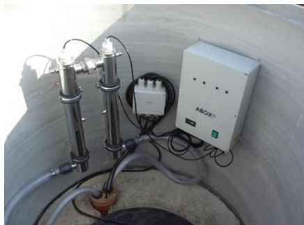
UV sterilisation of waste water
