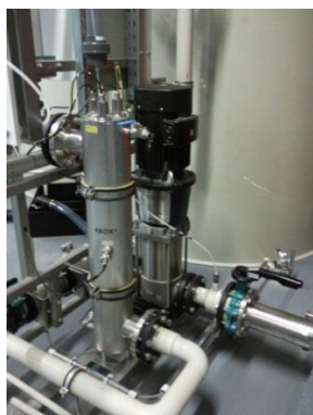
UV disinfection of process water
