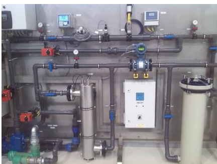
UV disinfection of process water
